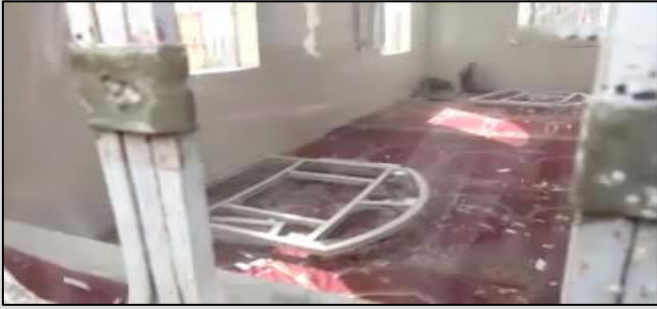
A photo of the mosque damaged by the airstrike
